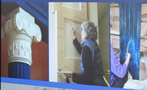
Restoration of gold and stone. Suzanne Collins and Elena Tucker Healdman restoring the original box finials on the doors and altar, respectively. faux finishes like these were not only very fashionable in the early 1800s, but also cost-effective. Courtesy of Historic Richmond
